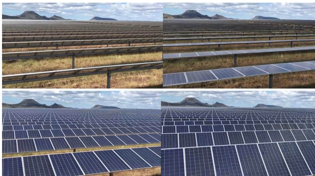
Figure 2-5: East-west single axis tracker system, finished array
