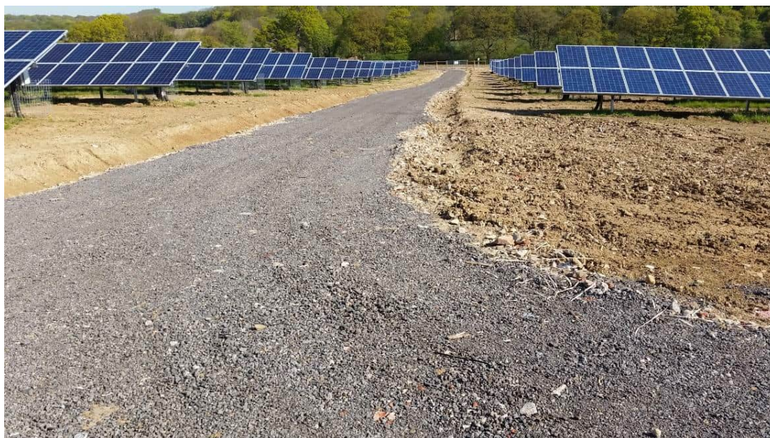
Figure 2-12: Typical crushed stone access track laid on hardcore and geotextile (photo during construction phase and prior to landscaping)
