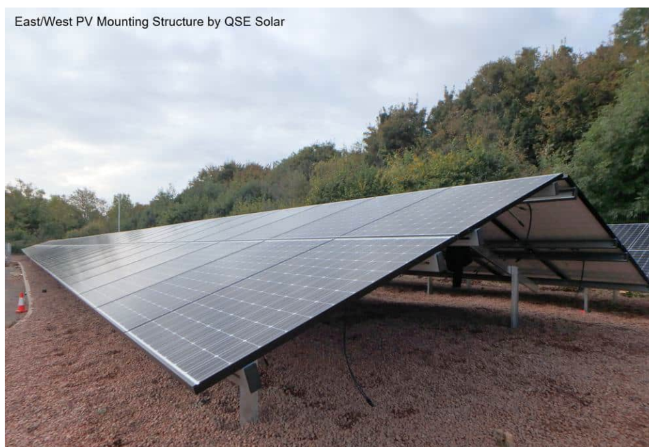
Figure 2-4: East-west facing fixed tilt modules, finished array
