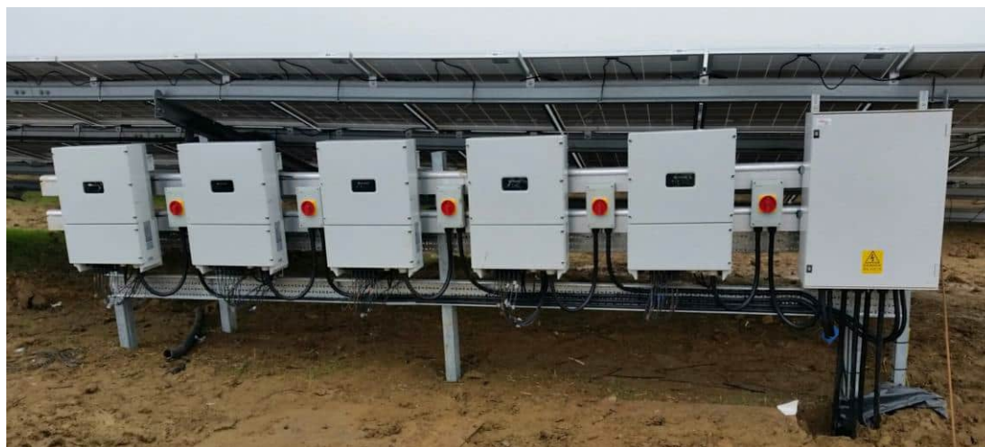
Figure 2-6: Typical string inverter installed under PV modules
